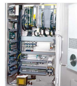
Electrical cabinet with heat exchanger.
